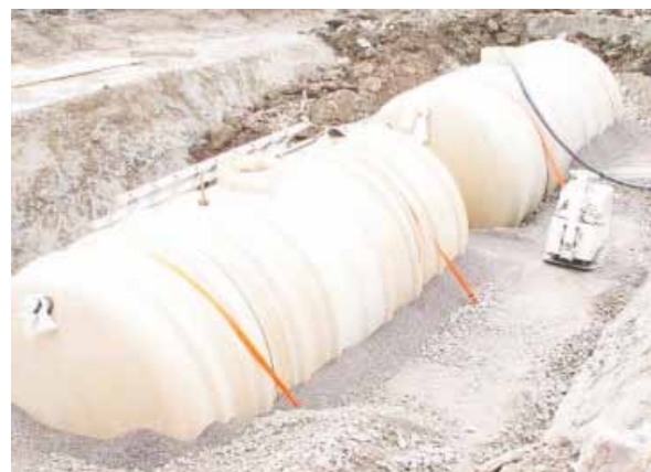
Figure 17: Storage tank during construction of housing area in Kullön, Sweden. Each tank is 12 m 3 .
